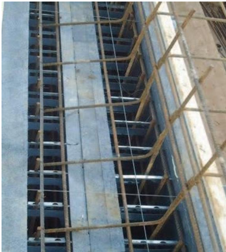
First Storey Basement Wall (650mm Double Wall) The second storey was erected with a single basement 350mm
