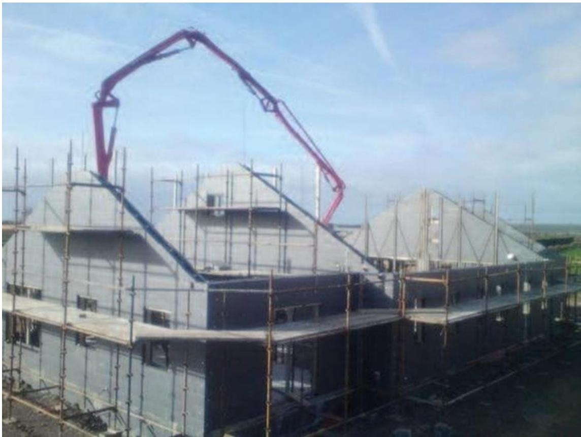
Single Concrete Pour To Full Wall Height - Floor To Ridge Level At 6.0m photo
