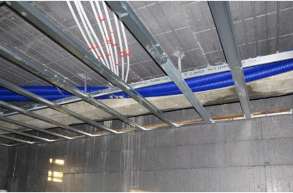
Suspended ceiling showing Services running in void
